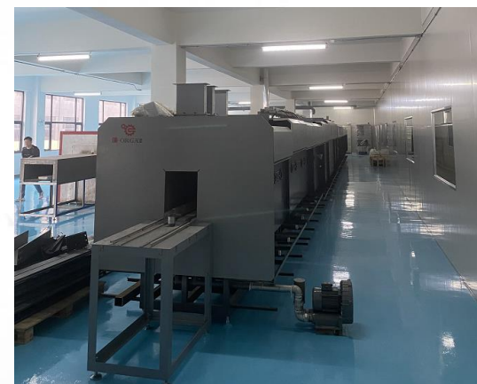
Degreasing sintering production line
